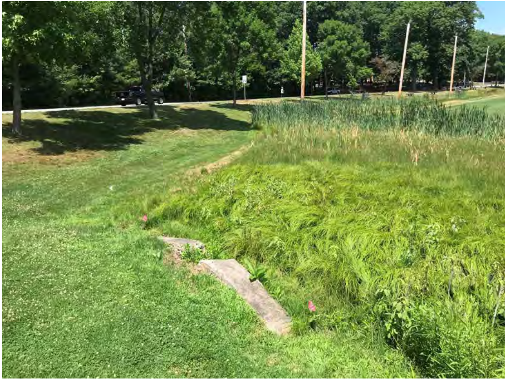
Photo 3: View of culvert outlet located in the northwest corner of the Study Area. Wetland vegetation is obvious from this view.
